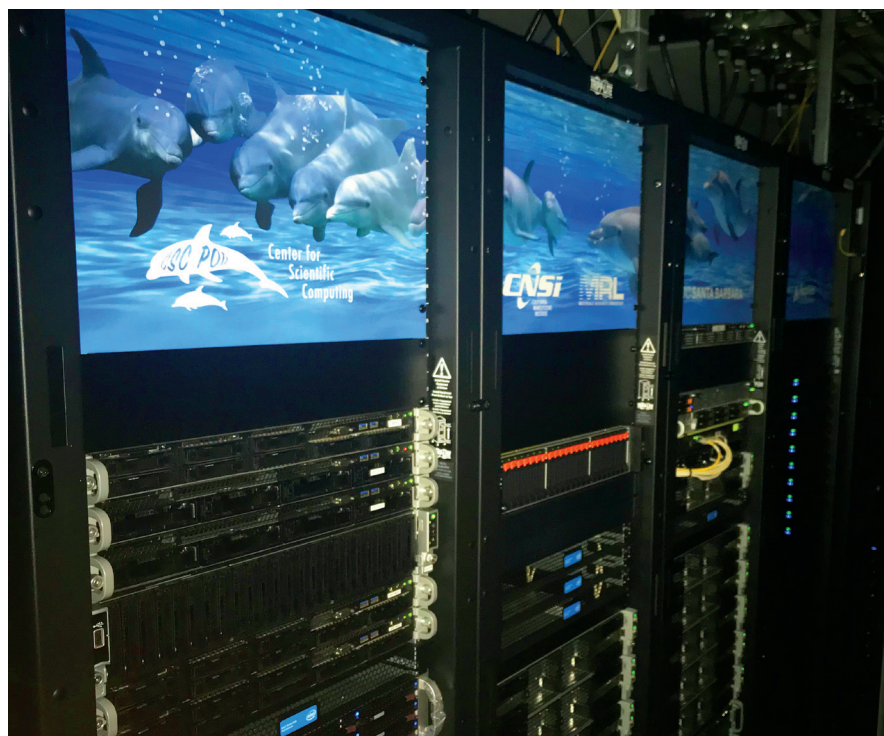
State-of-the-art nodes installed in the High Performance Computing campus cluster “Pod” in Elings Hall.
